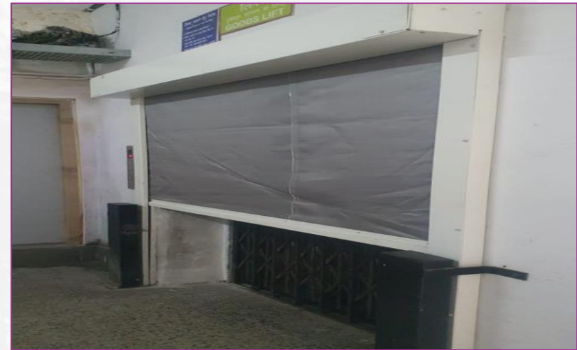
Panel room enclosure by fire door
