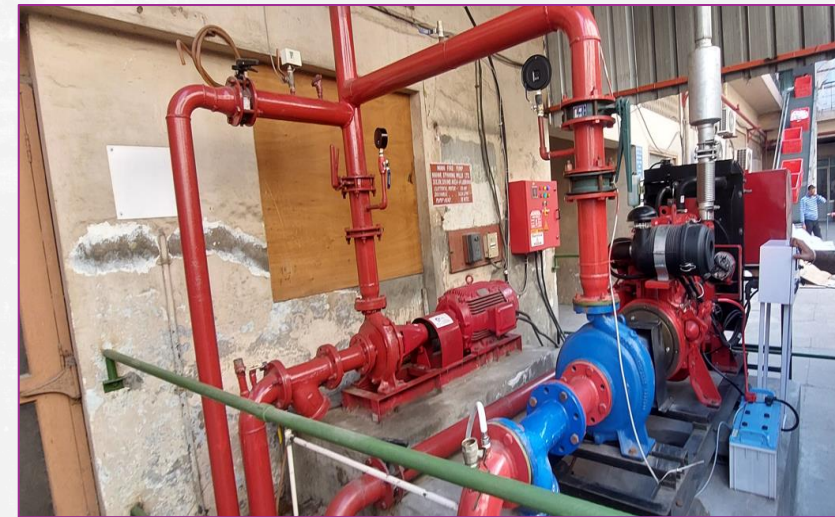
Backup Fire pumps are installed
