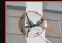
Crack in the pillar
