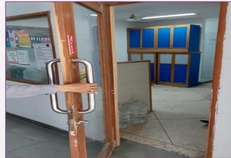
Rotating latch mechanism installed to bypass lock
