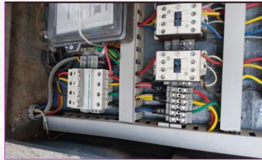
Electrical panel has been cleaned
