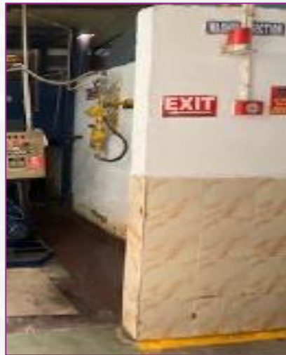
Visual hooters are added in utility area
