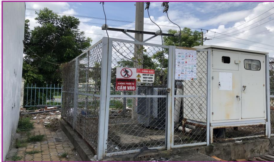
Sign age provided over substation
