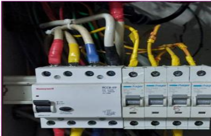
Lugs provided for electrical panel
