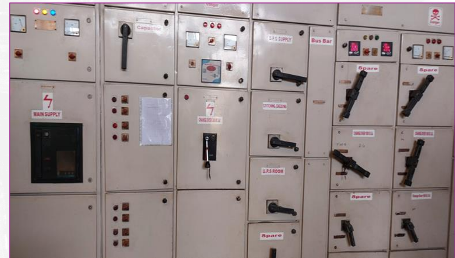
Proper identification provided over panel
