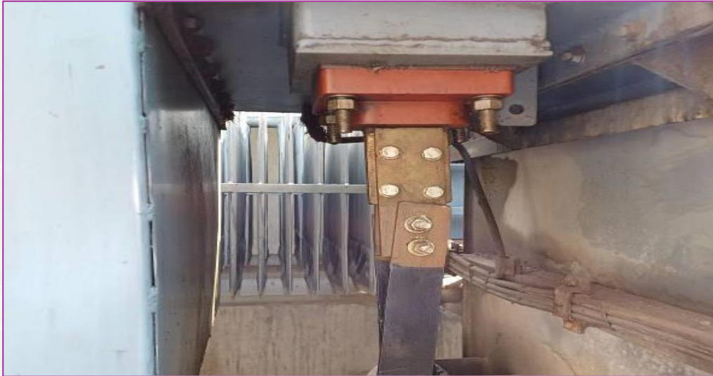
double Earthing provided to transformer
