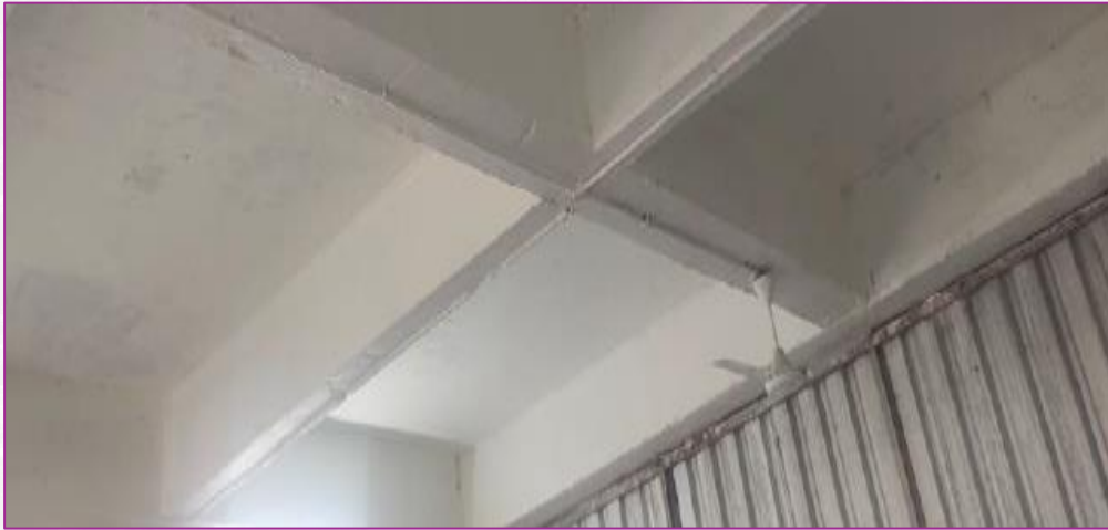
Dampness has been addressed
