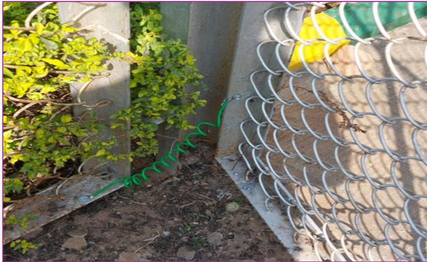
Bonding provided over transformer gate
