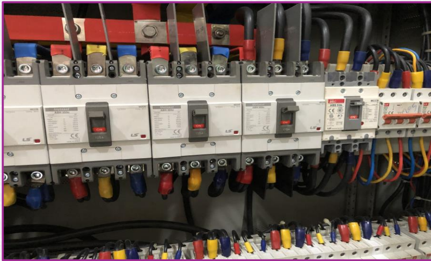
Electrical panel has been cleaned
