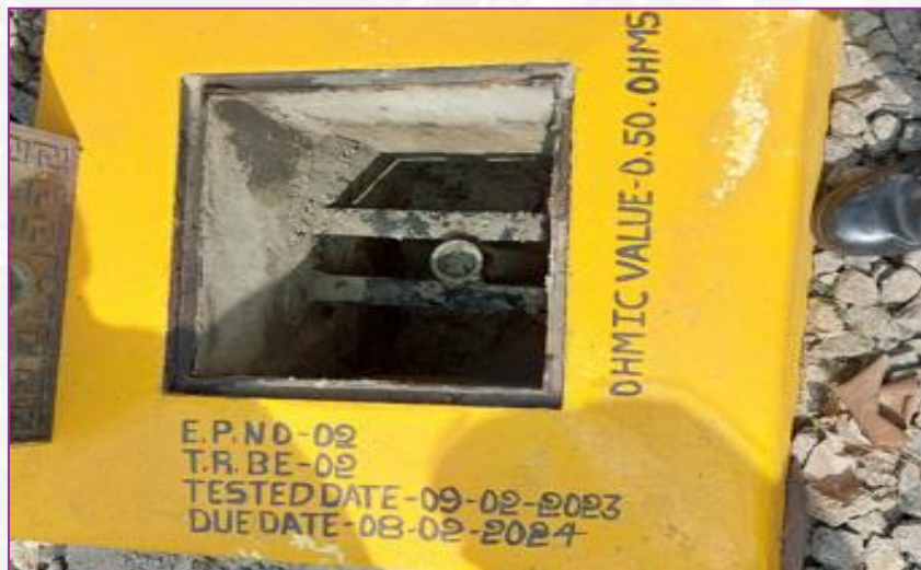
Earth pit maintained and monitored
