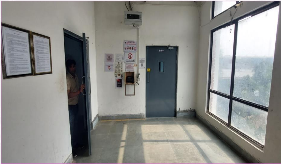
Staircase compartmentation with Fire doors
