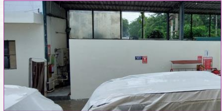
Wall separation provided between transformer & evacuation route
