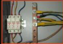
Multi looping of cables
