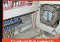
Combustible material inside electrical panel
