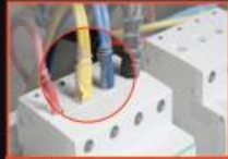
Lint/dirt on electrical panel
