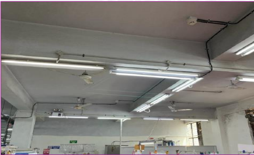
Smoke detector installed
