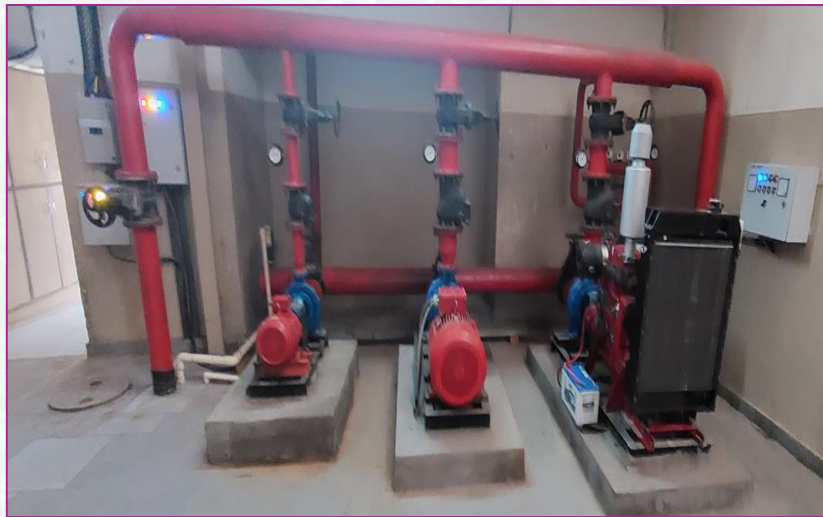
All 3 Fire pumps are installed
