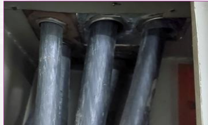
Glands provided over electrical panel
