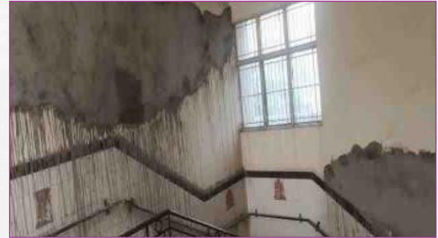
Dampness Repairs work has been done
