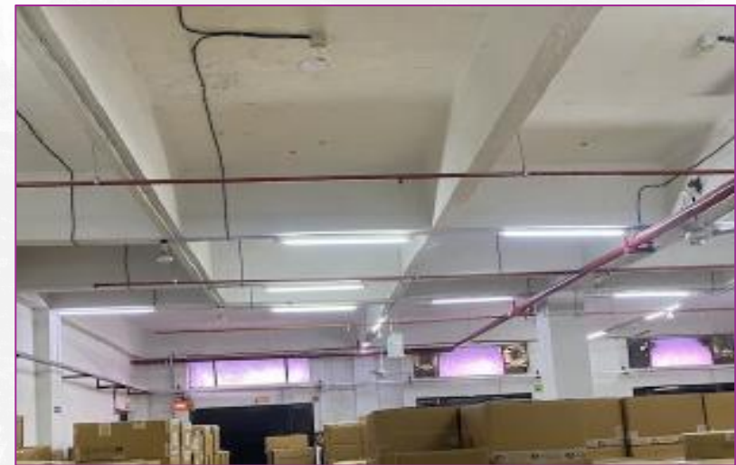
Sprinklers installed in material store
