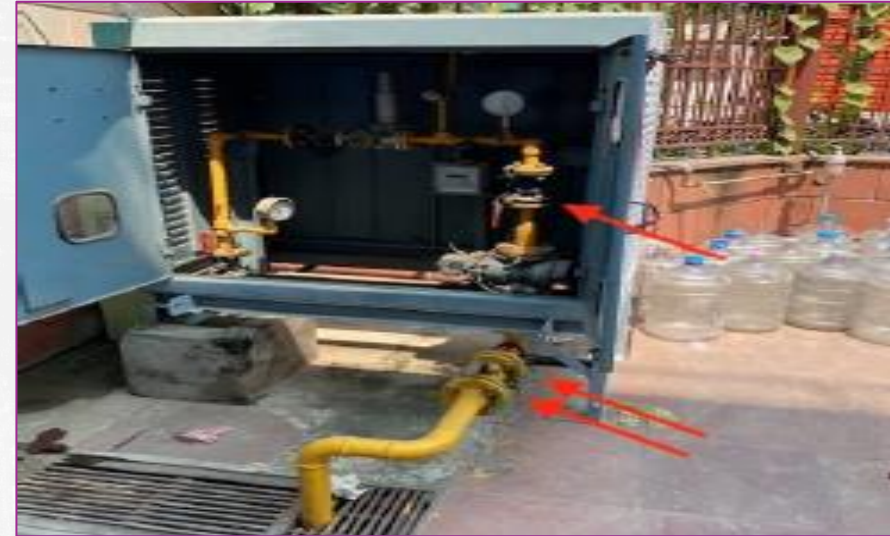
Bonding provided over LPG gas pipeline
