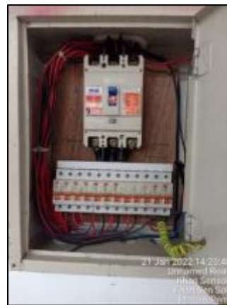
Figure 48: Combustible/flammable materials (wood) installed in SDB-0016B.
