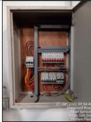
Figure 47: Combustible/flammable materials (wood) installed in SDB-001B.
