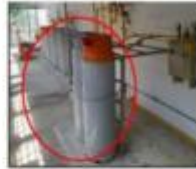
1.Over gas capacity storage behind building B.JPG
