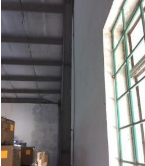
Figure N Bowing of masonry wall which is not restrained by steel columns in gable – c.30-40mm deflection at mid height of wall
