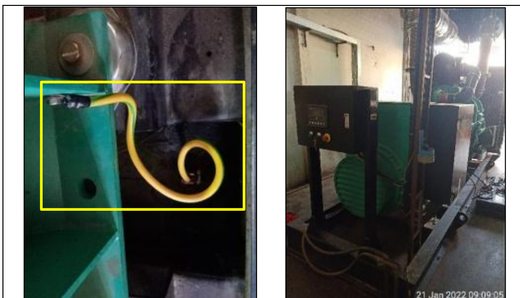
Figure 37: Insufficient generator 01 earthing with two separate points.
