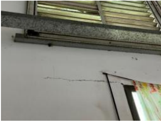
Figure 40: Wall cracking at building B
