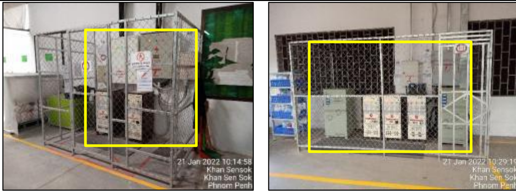
Figure 41: Insufficient Access to wall mounted DBs that blocked by floor standing Voltage Stabilizers.
