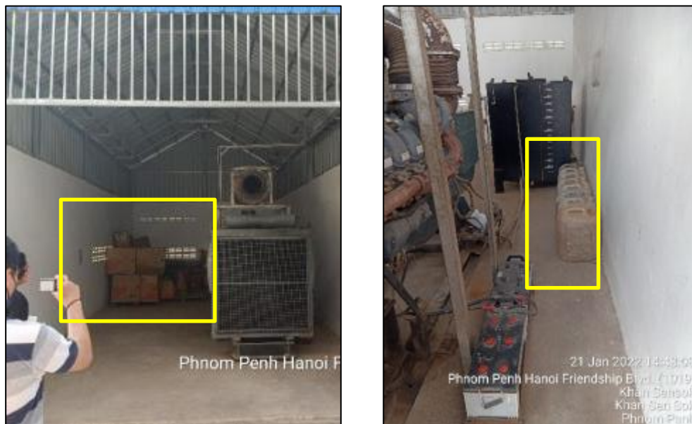
Figure 44: Combustible materials store inside generator room 02.
