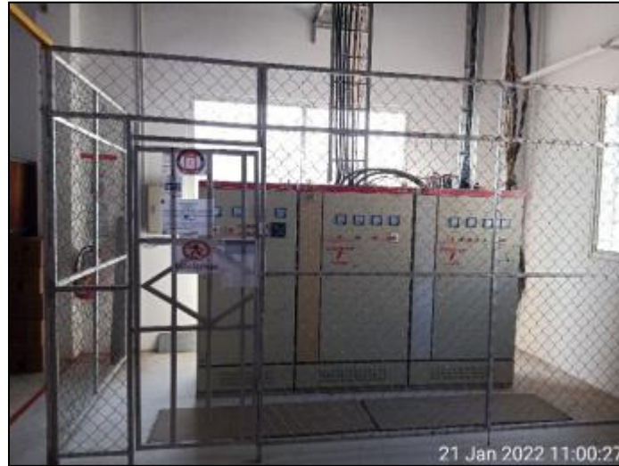
Figure 27: Main Distribution Boards (MDBs) inside Building C.
