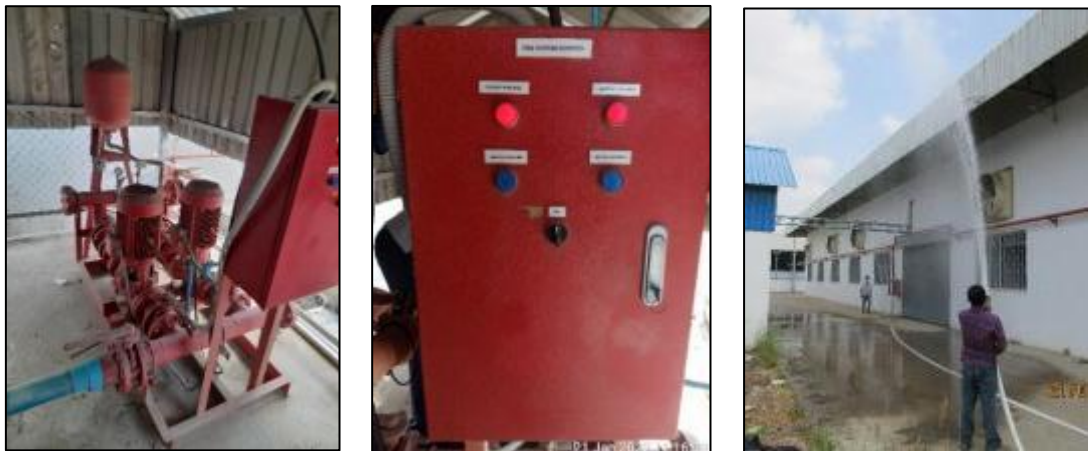
Figure 7: Fire Pump Station and Fire Hose testing
