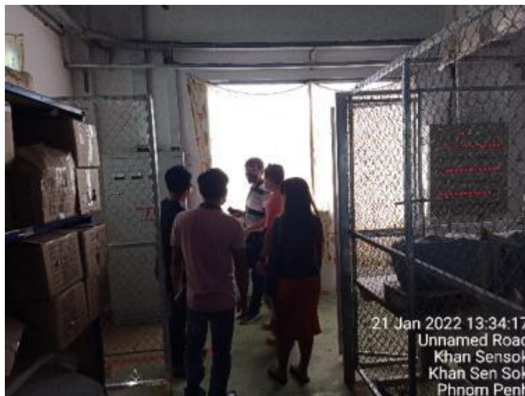
Figure 25: Distribution Boards (DBs) inside building B.
