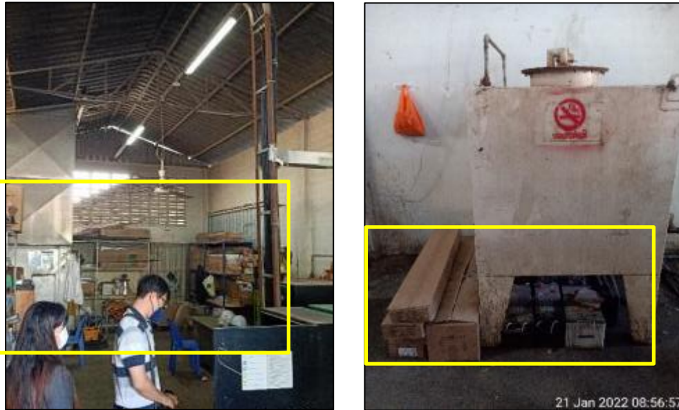
Figure 43: Combustible materials store inside generator room 01.
