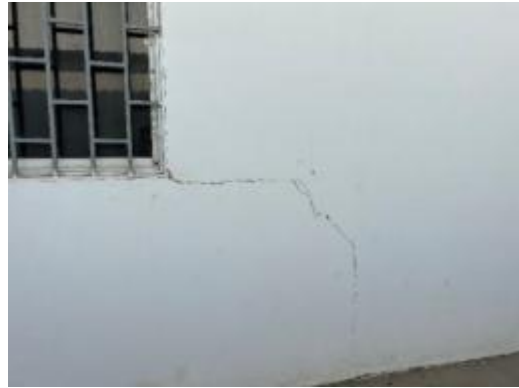
Figure 43: Wall cracking at building C
