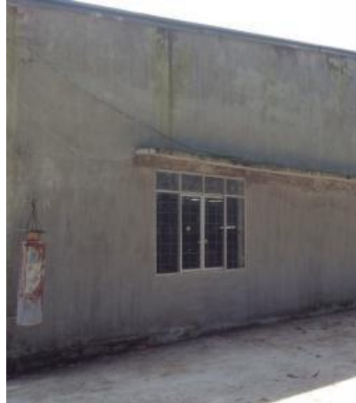
Figure N View of northern gable wall with apparent repairs / new render. Concrete canopy appears to have deflected
