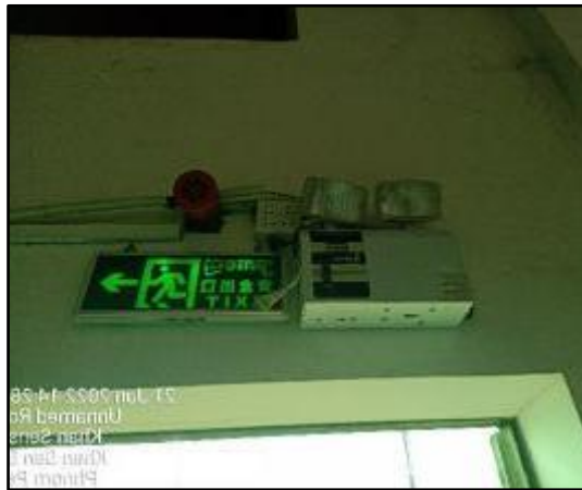
Figure 10: Inadequate back up power to emergency lighting
