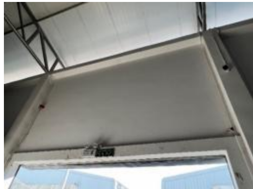
Figure 41: Wall cracking at building C
