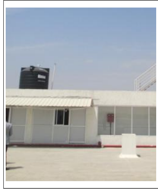
Figure N 10,000 liters tank at GL 0-11/D-E
