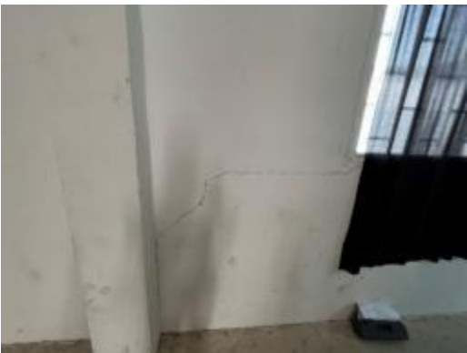
Figure 42: Wall cracking at building C
