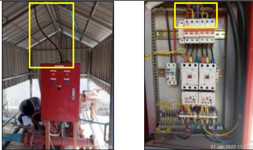
Figure 57: Normal insulation power cables from MDB in Building A to FF pump control panel.
