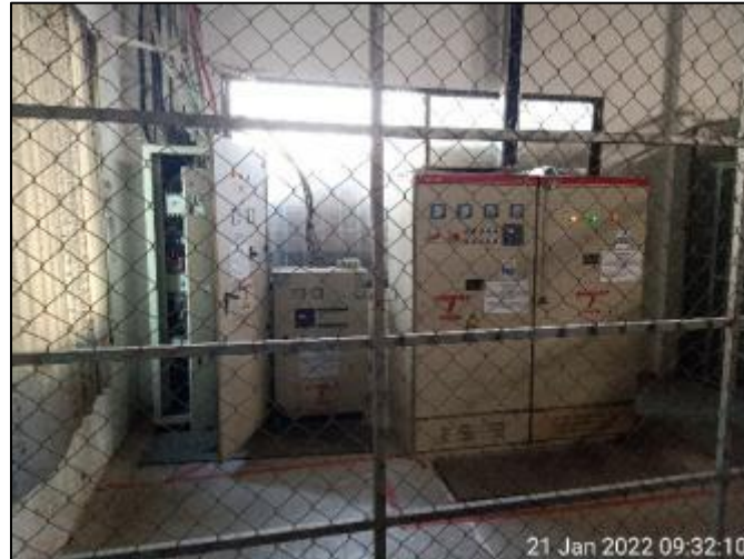
Figure 22: Main Distribution Boards (MDBs) insides building A.
