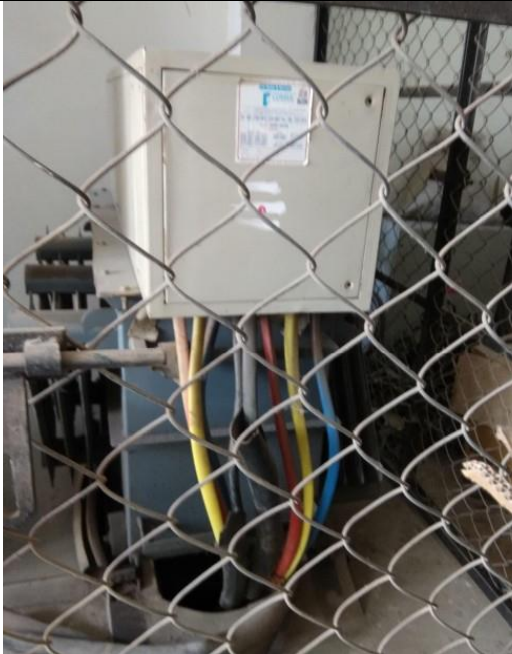
Figure N Improper termination of cables.
