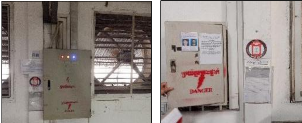
Figure 24: Sub Distribution Boards (SDBs) inside building A.
