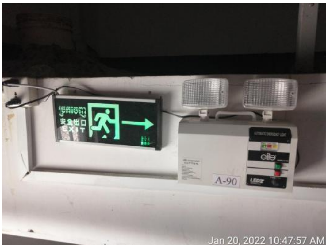
Figure N Emergency Lighting
