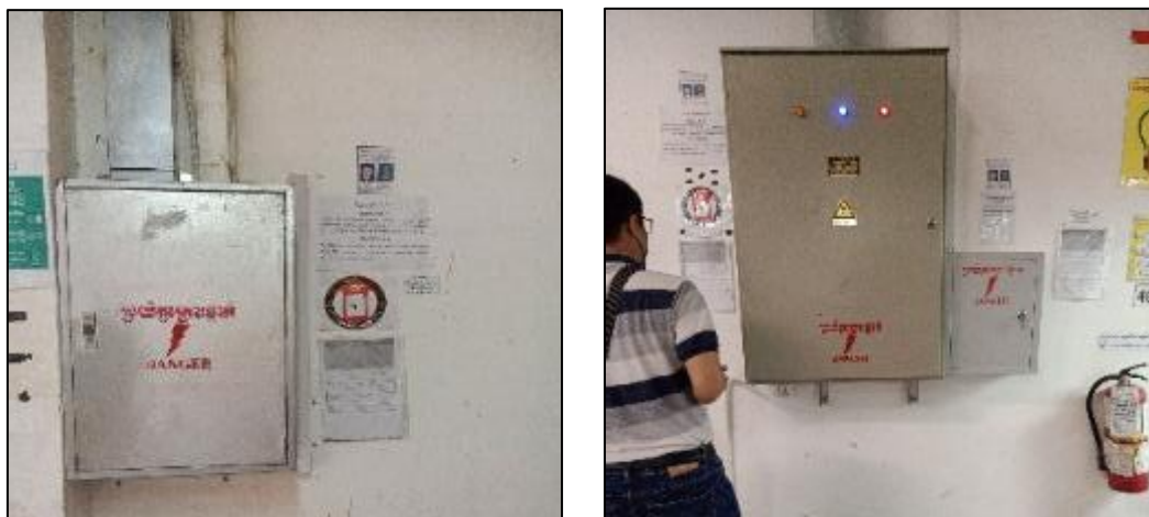
Figure 26: Sub-Distribution Boards (SDBs) inside Building B.
