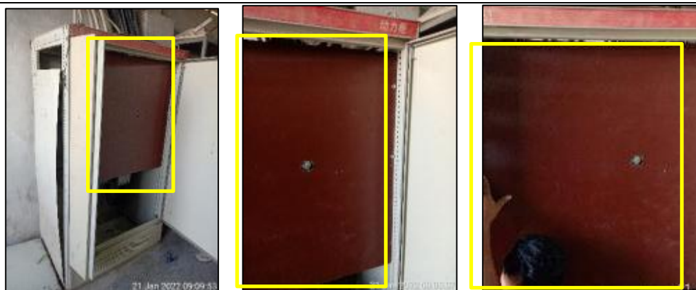
Figure 42: Panels cover damaged and replaced with unsafe flash guard when need to open to the LVMSB/MTS 01 & 02 cover.
