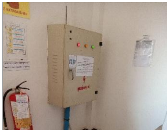
Figure 28: Distribution Board (DB) inside Hostel Building.
