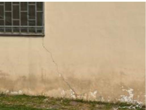
Figure 44: Wall cracking at Hostel building
