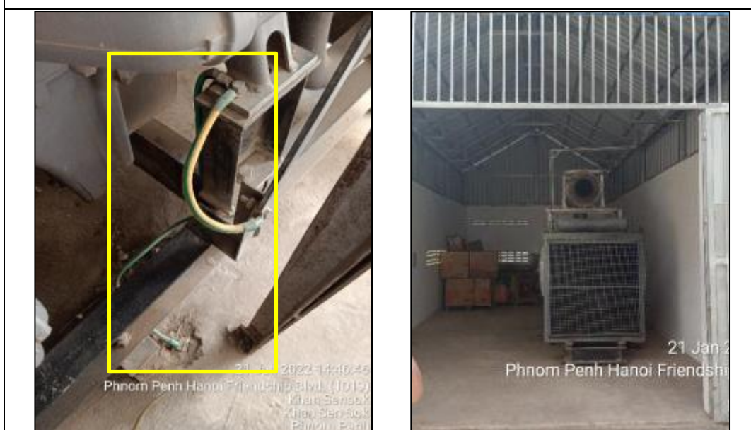
Figure 38: Insufficient generator 02 earthing with two separate points.
