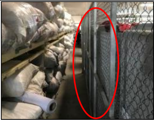
Figure 29: Separation of different occupancies was incomplete between storage area at building B
