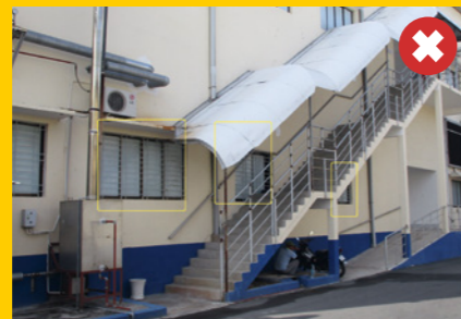
No fire rated enclosure for external staircase
