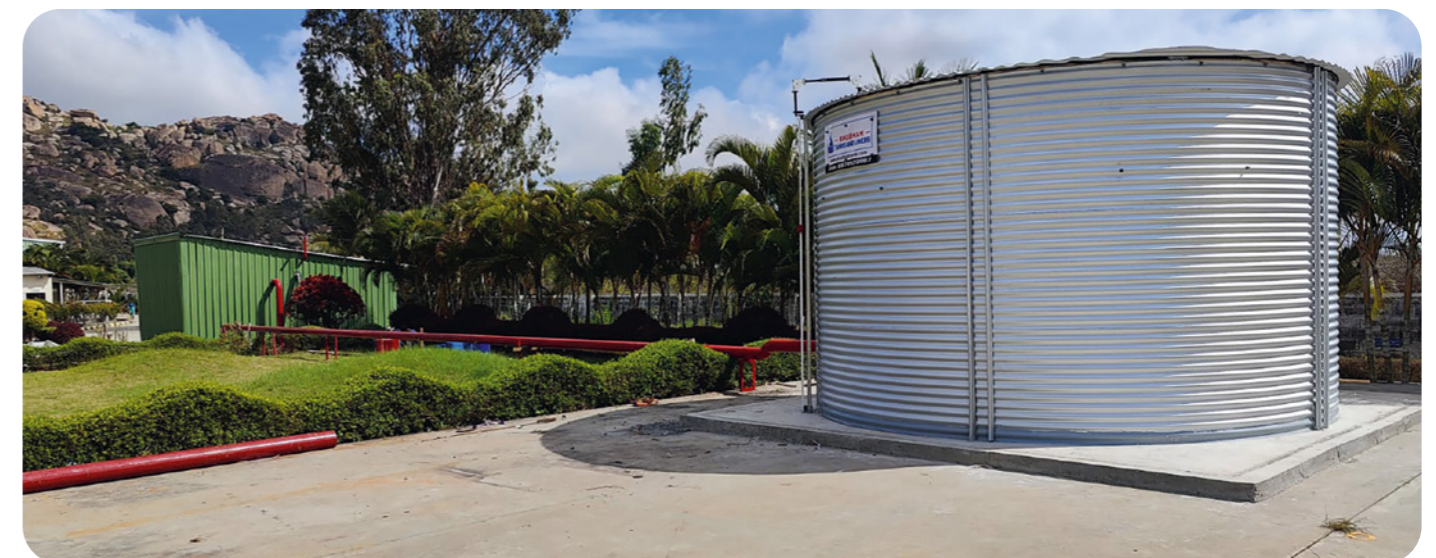
Fire water tank installed as a part of remediation at one of the LABS-assessed factories
