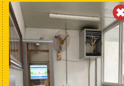
Fire detection not installed
