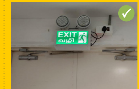
Illuminated exit sign provided over emergency exit
