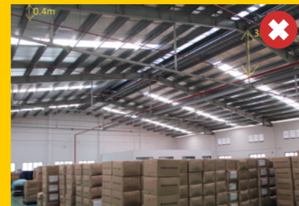
Sprinkler system installed far beneath the ceiling
