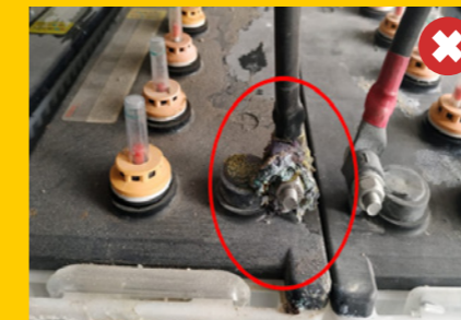
Exposed battery terminals
