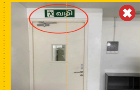
Illuminated exit sign not provided over exit
