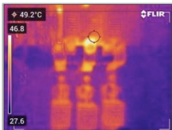
After - Temperature noted - 49.2°C
